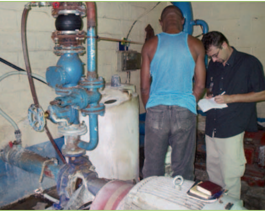
Audit of a chlorination plant in cooperation with REGIDESO
